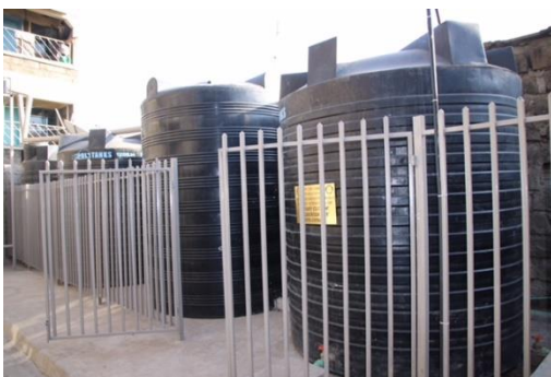
New water system for school.
